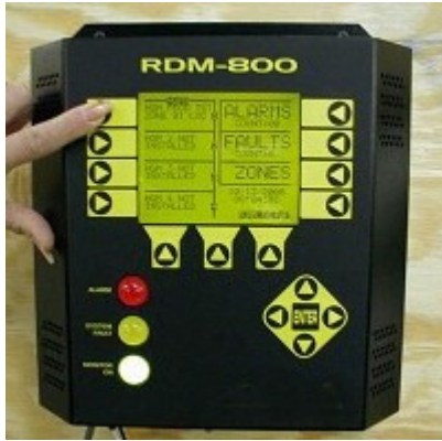
Figure 5. Push button of monitor being serviced to display its SETUP Screen
